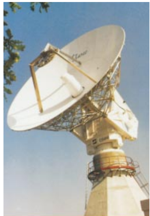
Figure 12-17: A typical, but large telemetry reception antenna.
