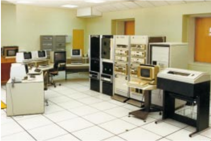
Figure 12-18: Representative ground-site telemetry receiving and processing equipment.
