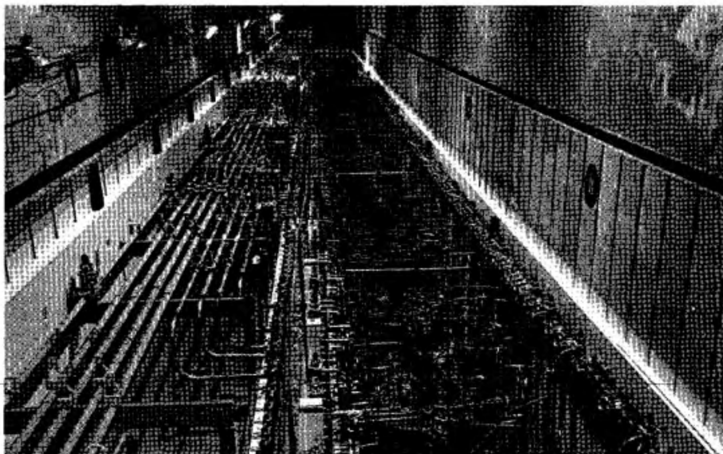
Figure 74 Warm Canyon Interior One of the Chemical Separations Facilities at SRP prior to startup.
